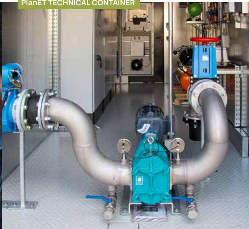
PlanET TECHNICAL CONTAINER
