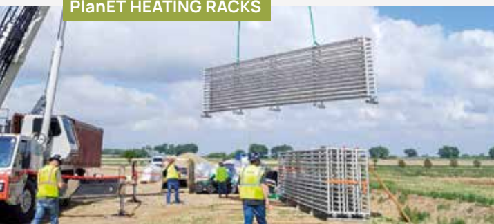
PlanET HEATING RACKS
