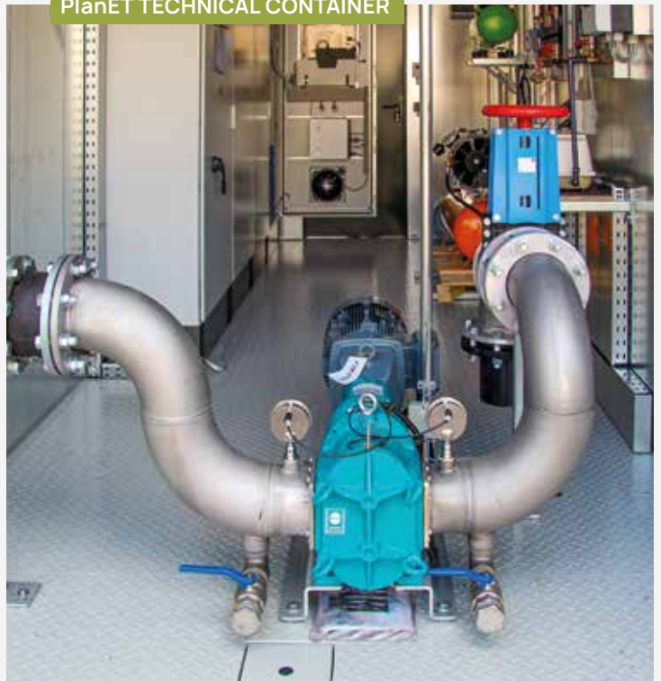
PlanET TECHNICAL CONTAINER
