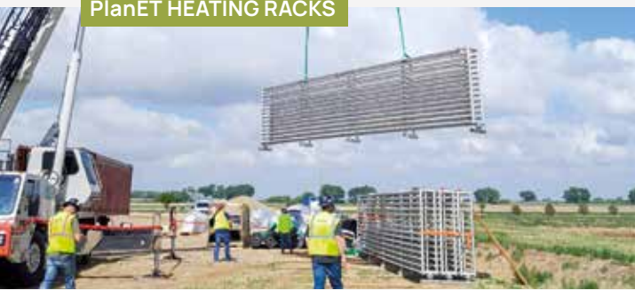
PlanET HEATING RACKS
