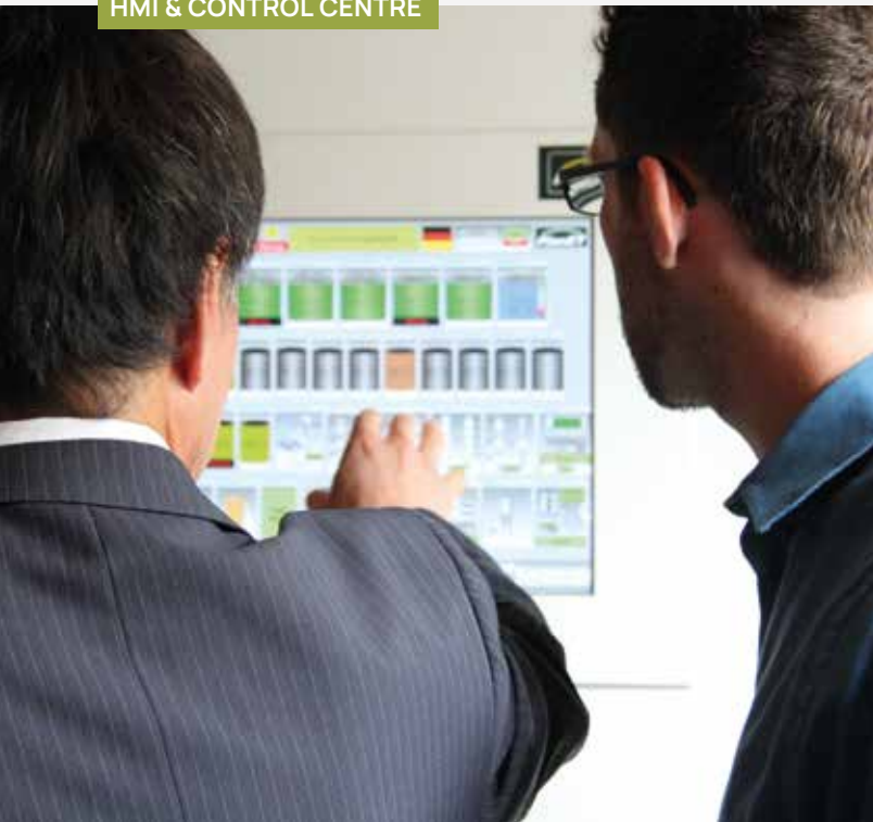
HMI & CONTROL CENTRE
