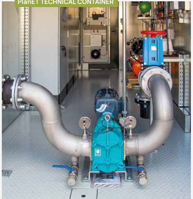
PlanET TECHNICAL CONTAINER
